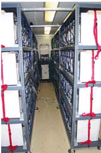
Figure 3. 156 Dual-Processor PC Cluster. The boxes are connected using a standard 100Mbps Fast Ethernet network (the green and blue cables). In the back, one can see the 192-port Cisco switch. The height of the shelving system is approximately eight feet.
